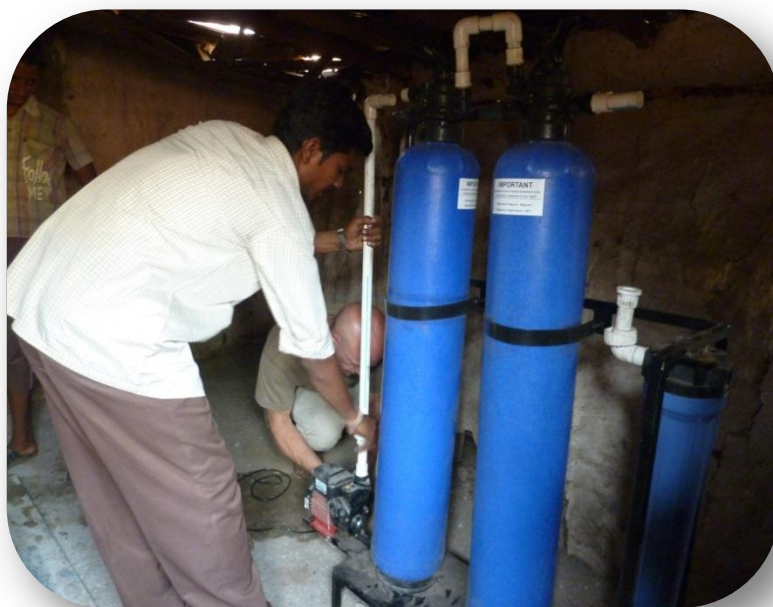
Installation of the New Water Filter
