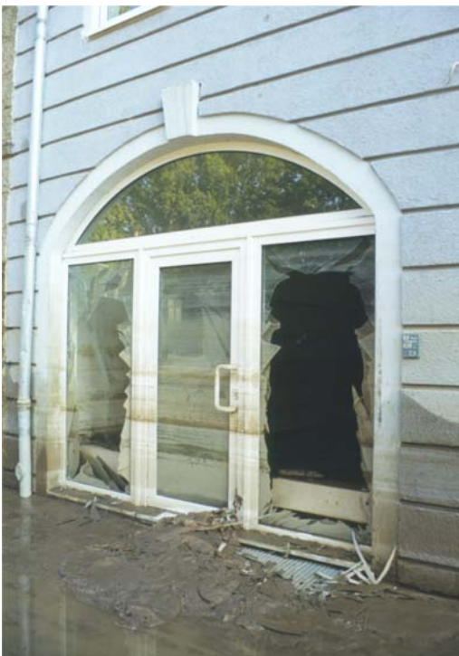
Collapse of glass-fronted office. The water level in this street reached ~1m above ground level.
